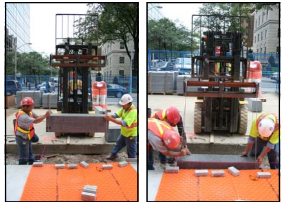
Above, construction workers install the first piece of granite curb in front of St. Paul's Square on Sept. 29 th .
